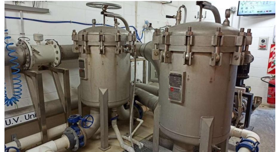
Figure 10 - Water filtration system at Kaipaitangata water treatment plant
