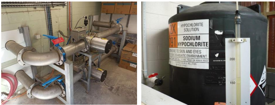
Figure 9 – Carterton’s water disinfection systems
