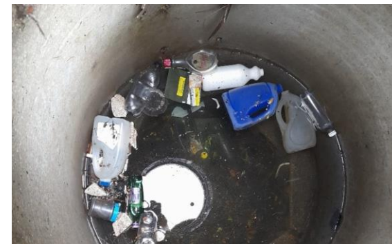
Figure 18 – Debris found in the wastewater network
