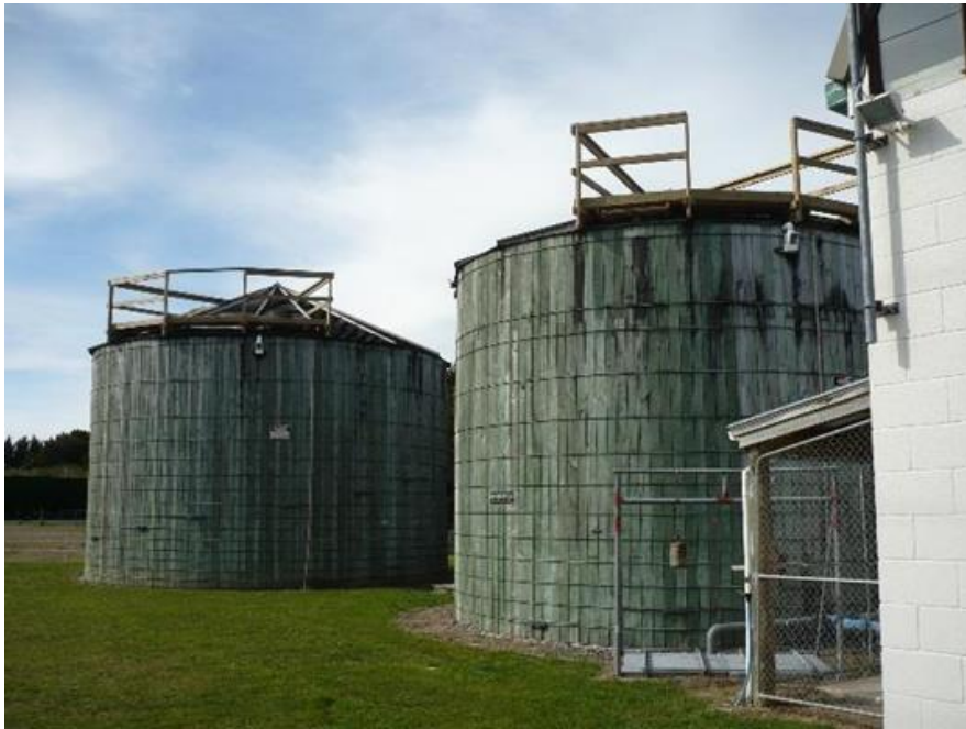
Figure 6 - Lincoln Road water storage tanks
