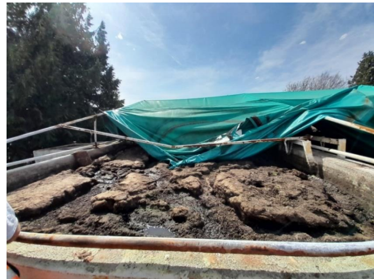
Figure 15 - Sludge dewatering facility at Dalefield Road wastewater treatment plant
