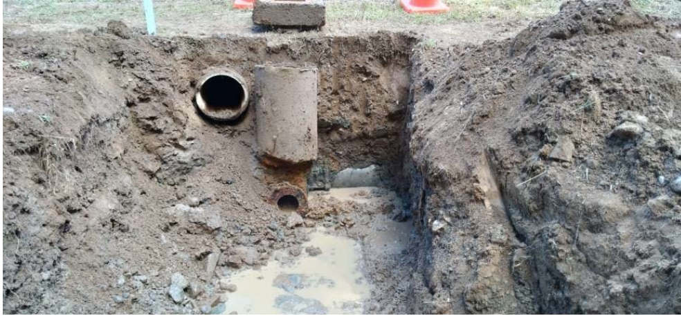
Figure 3: A view of the culvert (top left) and the scour valve visible at the base of the trench.
