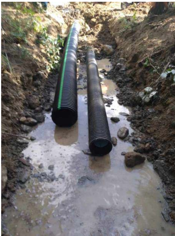
Figure 4: Pipe extension attached to both the culvert and replaced scour valve outlet.
