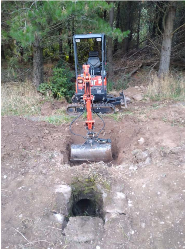
Figure 2: The foreground shows the culvert sump with the outlet of the culvert seen in the picture.
