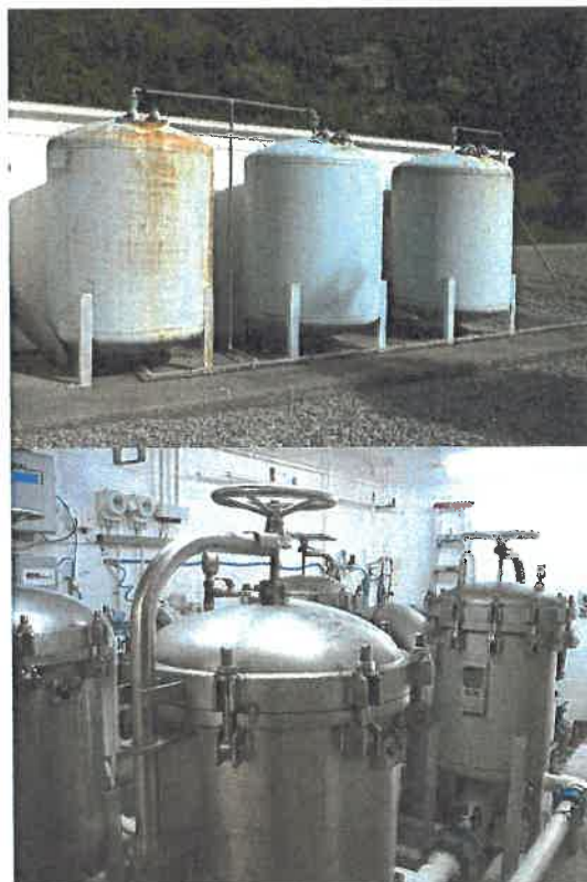
Pressure media filters (left) and bag filters (right)
