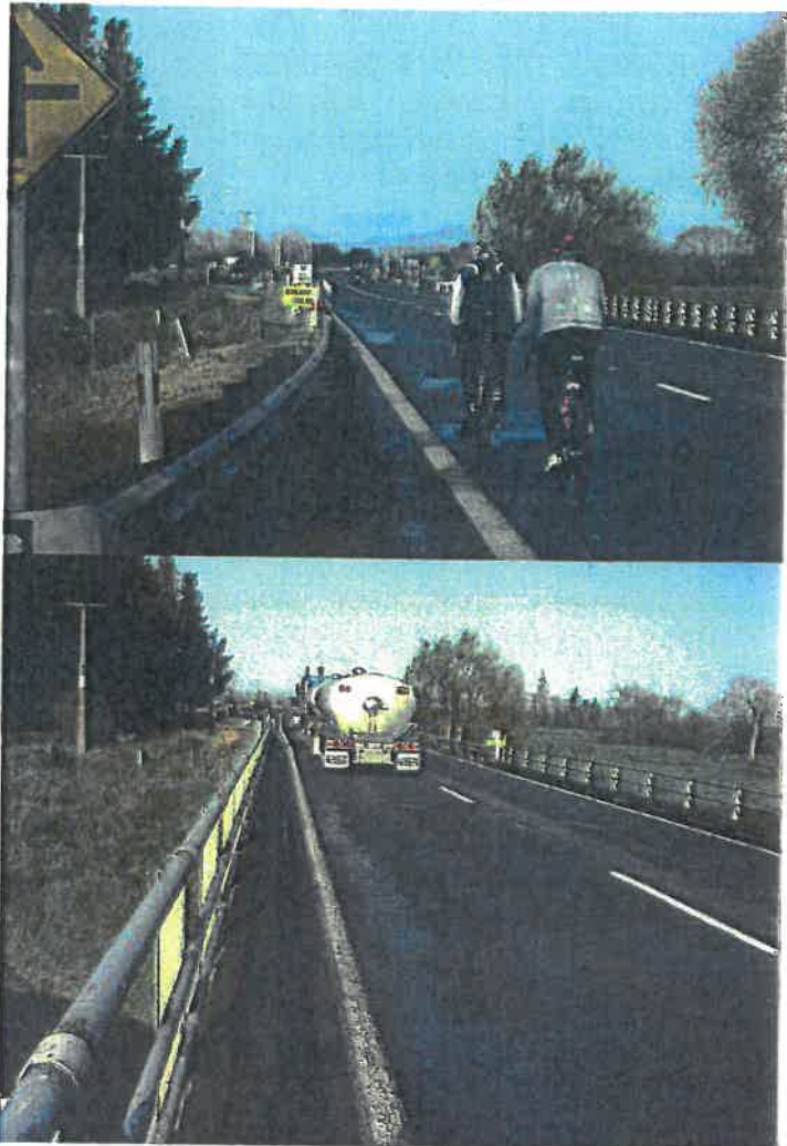
Kaipaitangata Stream Bridge, State highway 2, near Carterton's western boundary with South Wairarapa District. The lower photograph was taken a few seconds after the upper one.
